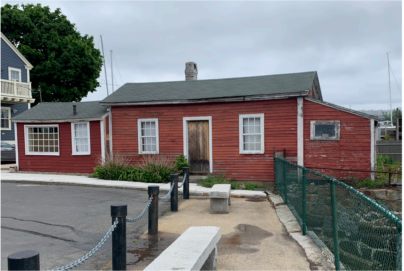
The exterior of the Primm House, showing deterioration and settling. Interior evaluation was not part of project scope. Photo by Union Studio.
