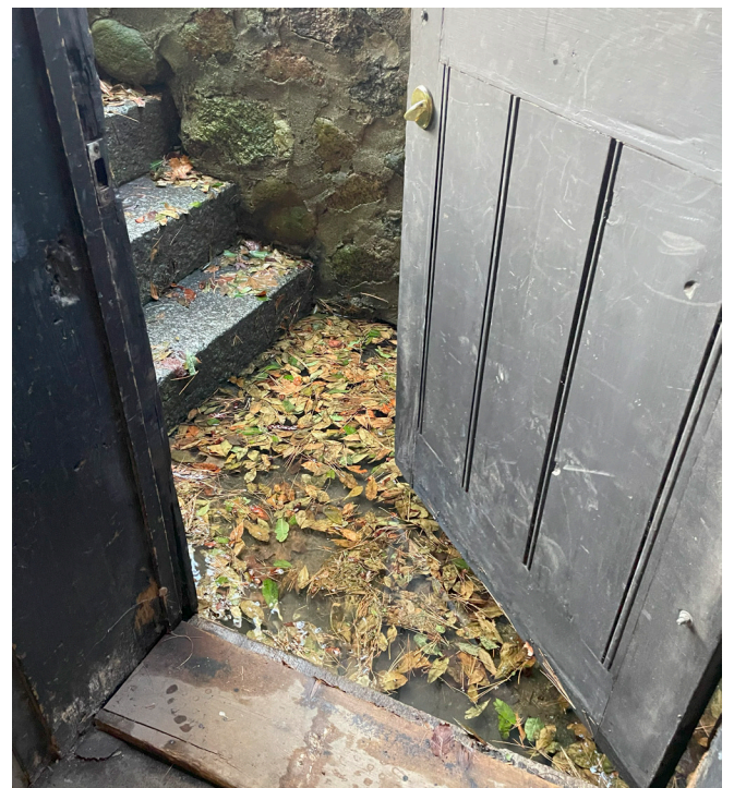
The basement stairwell flooding during a storm event, 1/10/24. Photo by the House of the Seven Gables.
